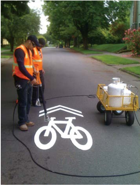
Figure 48 | Communities with paved roads need not wait for road reconstruction to incorporate bicycle facilities. Adding shared lane markings (sharrows) is a feasible, budget set aside project that will work well in many situations. Photo credit: Oregonlive.com
