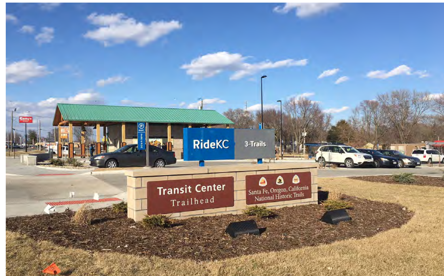
3-Trails Transit Center at Blue Ridge Blvd and Bannister Rd (connecting to segments 21c and 21d) under construction, Dec. 2017. Photo: M. Graf
