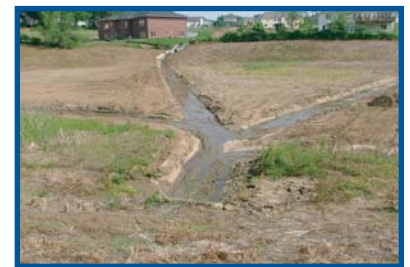
One aspect of the project involves the stabilization of silt in the concrete channels.
