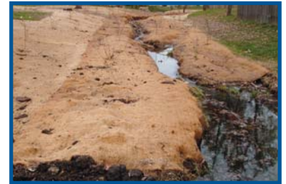
This upstream shot of the Harmony Park project demonstrates the use of erosion control blankets and native plantings.
