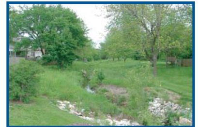
Downstream, the overflow plane has been graded back to allow greater capacity in large rain events while rock grade controls provide streambed protection.
