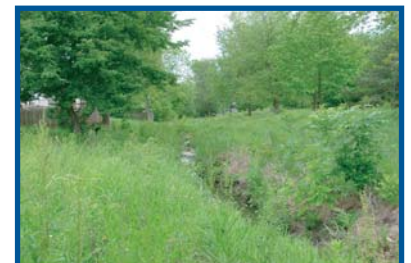
Plantings of native vegetation reinforce the streambank protection provided by the erosion control blanket.
