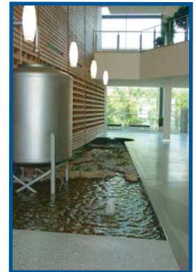
Interior water garden filters runoff from the building's roof.
