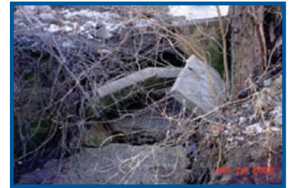
Complete erosion of the concrete aprons in the Lazy Branch Creek.
