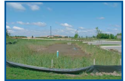
Bioretention cells with native vegetation are positioned to filter runoff from the parking lot.
