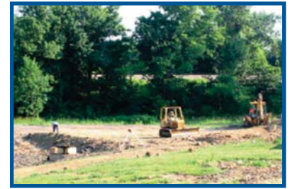
Construction of the wetland will mitigate excess water flows into Sni-a-bar Creek.
