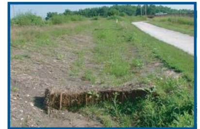
Conversion of an eroding ditch to a vegetated swale provides improved stability and aesthetics.
