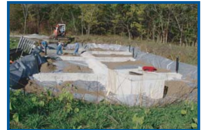
The bioretention system consists of several materials designed and sized to maximize water filtration and plant growth.
