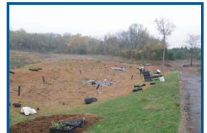
The bioretention soil mixture is covered by a 3-inch layer of mulch and nearly 5,000 plants.
