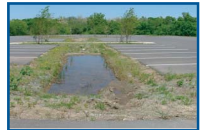
Drainage issues have been a major problem for the bioswales.
