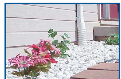
Stormwater is collected at the downspouts
