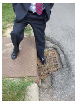
Hazardous sewer grates
