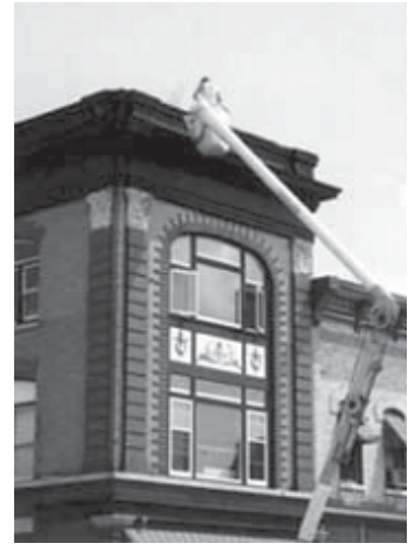
Upper Façade restoration in progress on the Erickson Building in Downtown Stoughton ( www.silberschmidtdental.com/office.htm )
