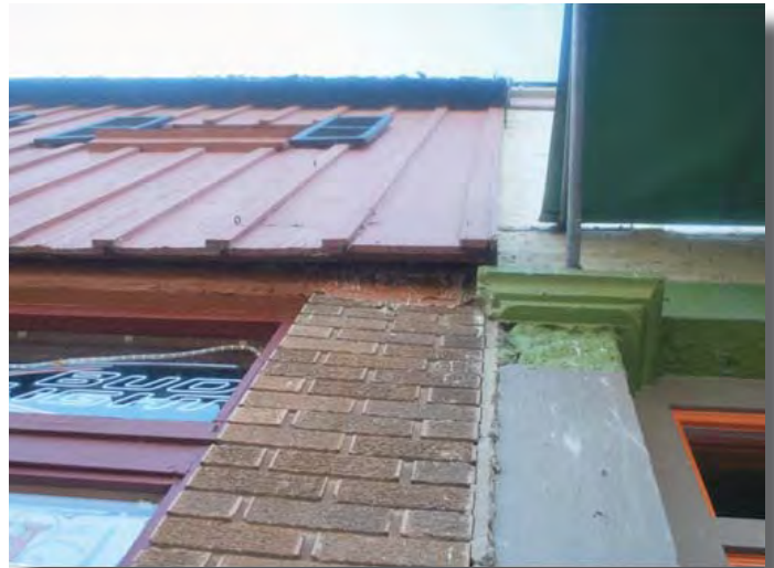
Fig. F.25 – View of the gap between the wood board and batten siding which has been installed over a layer of stucco which has been applied to the upper half of the masonry façade. (SRJA, 2013).
