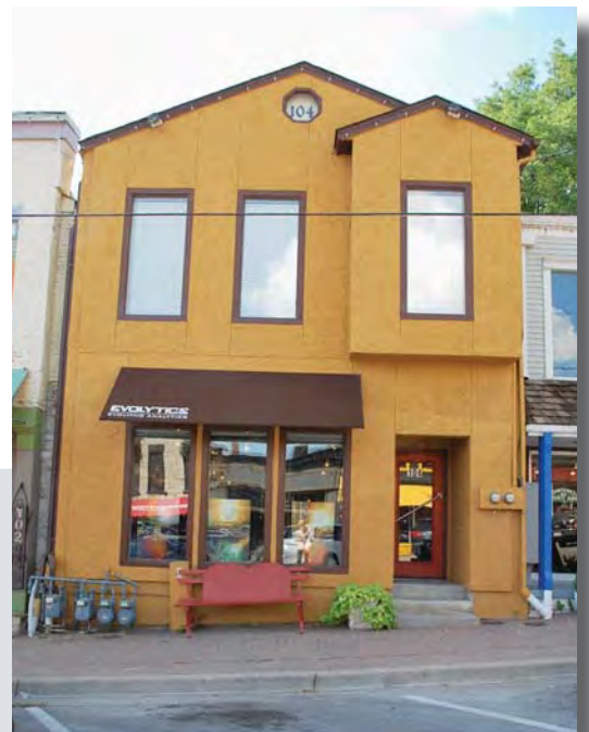
Fig. F.29 – View of stucco system known as EFIS which has a layer of rigid foam insulation which has been applied to the exterior of the building. If the stucco layer is removed, the historic building façade could be restored. (SRJA, 2013)
