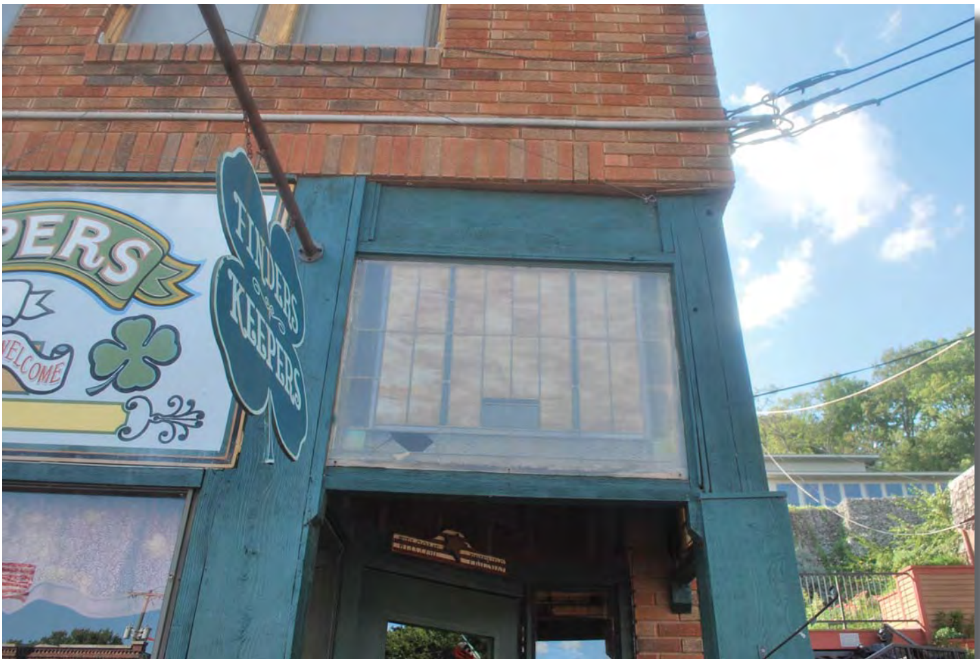
Fig. F.4 – View of faded painted signs and stained glass transom window with a deteriorated, filmy protective glazing and trim. (SRJA, 2013).
