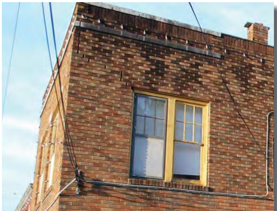
Fig. F.24 – View of a masonry wall in need of repointing and cleaning. Note the cracked mortar and bricks extending from the left corner of the window up to the corner of the parapet. (SRJA, 2013).
