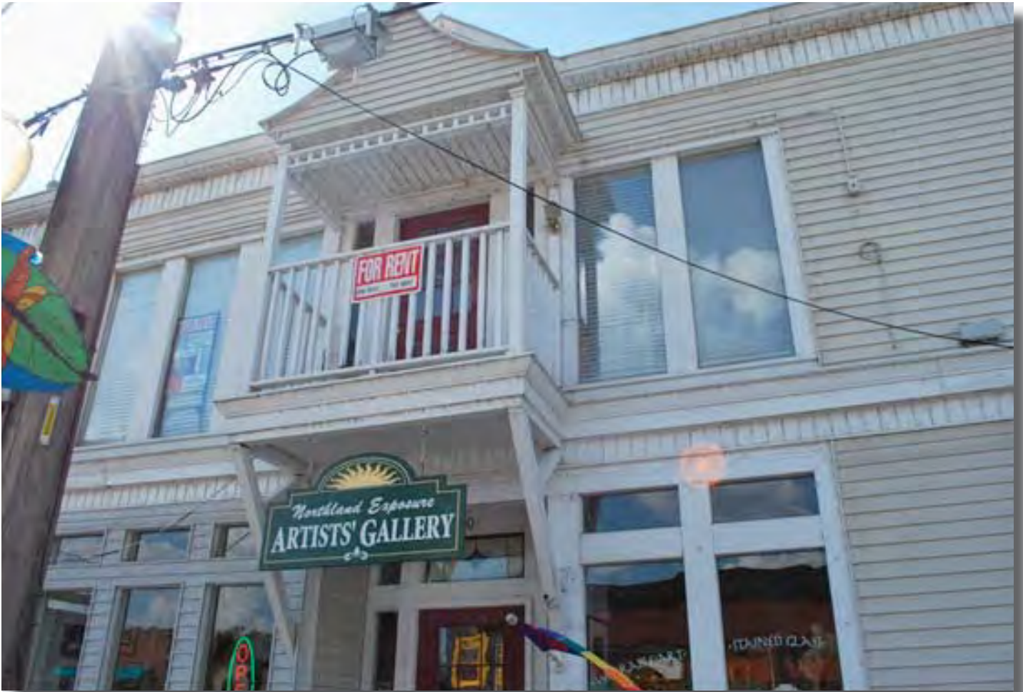
Fig. F.26 – View of vinyl siding applied to the exterior of a building. The vinyl siding is dirty and has evidence of vines which grew across the entire façade at one time. (SRJA, 2013).
