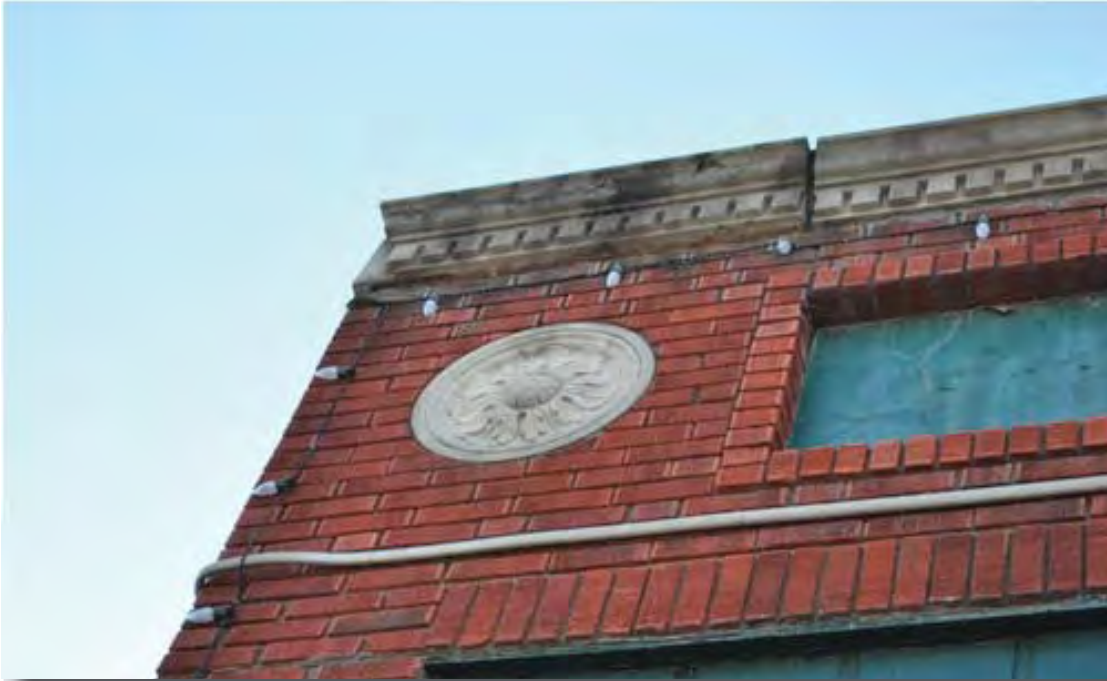
Fig. F.23 – View of dirty stone cornice with open mortar joints in need of repointing. (SRJA, 2013).
