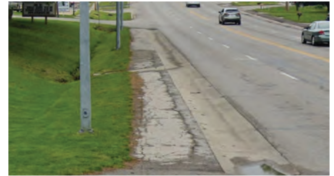
FIGURE 4.1 - DRAINAGE DITCHES ON NORTH OAK BETWEEN BRIARCLIFF AND I-29 WILL REQUIRE ADDITIONAL CONSIDERATION
