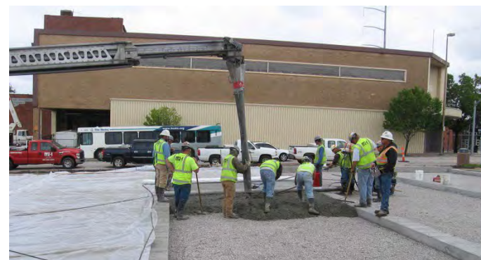
Figure 46: Porous concrete paving effectively manages stormwater runoff.
