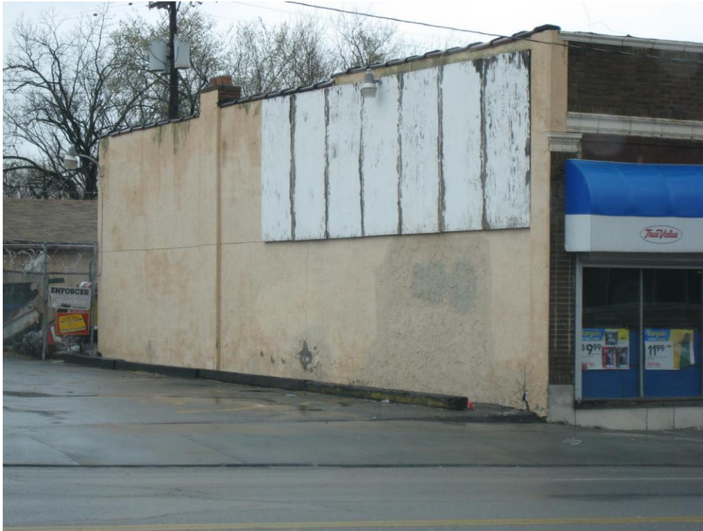
Deteriorated exterior walls and paint on north side of 4627 Troost Avenue (Deteriorated or inadequate site improvements)
