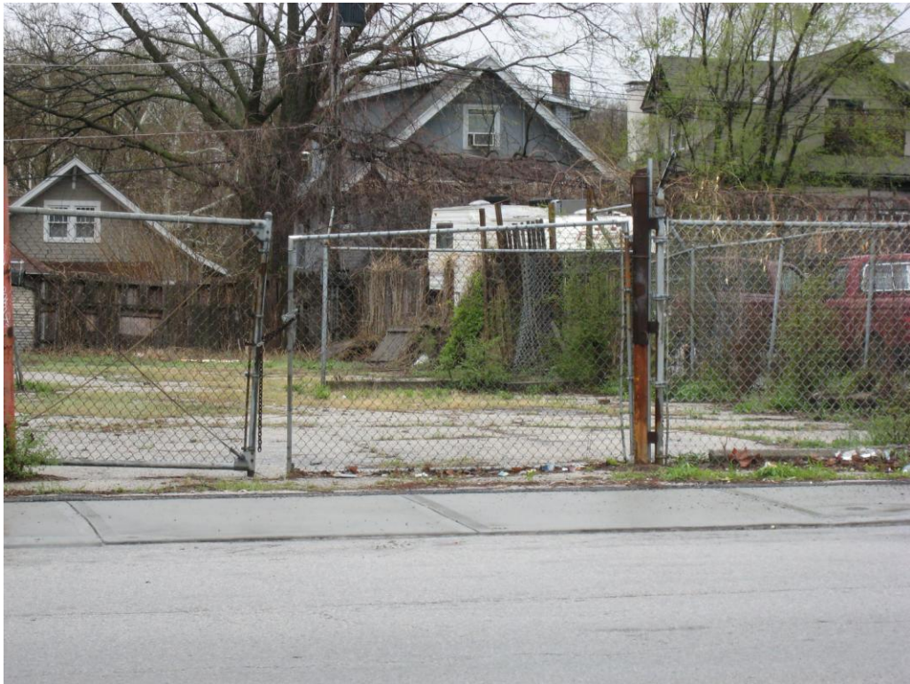
Deteriorated fencing and site conditions of vacant parcel at 4512B Troost Avenue (Deteriorated or inadequate site improvements, Economic and social liability)
