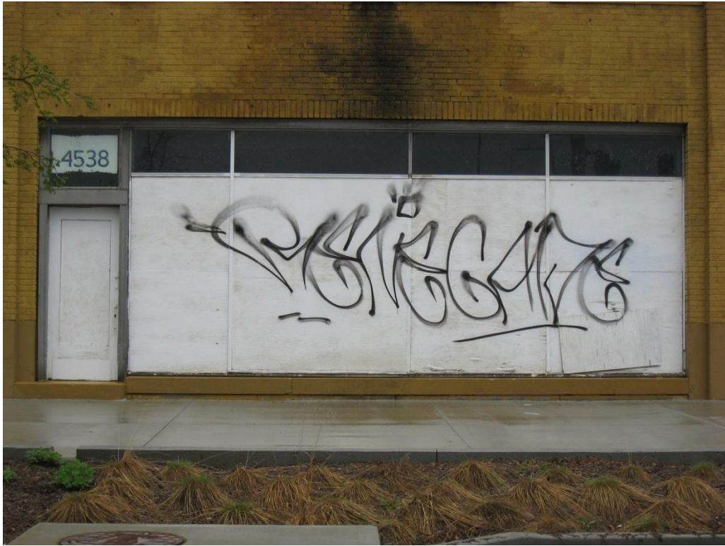
Deteriorated exterior wall conditions and graffiti at 4538 Troost Avenue (Deteriorated or inadequate site improvements, Menace to public health, safety)
