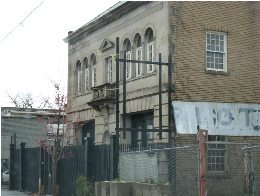
Deteriorated site conditions, vacant historic building at 4518 Troost Avenue (Deteriorated or inadequate site improvements, Economic and social liability)
