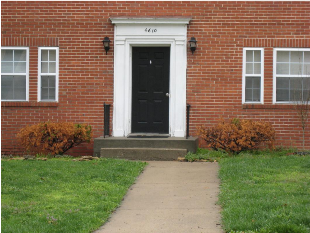
Lack of accessible route and primary building entry at 4610 Campbell Street (Unsanitary and unsafe conditions)
