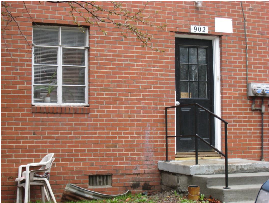
Indications of poor maintenance at rear of property at 902 Emanuel Cleaver II (Deteriorated or inadequate site improvements, Menace to public health, safety)
