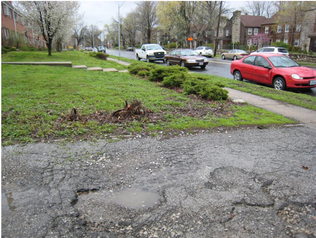
Deteriorated site conditions southeast corner of property at 4616 Harrison (Deteriorated or inadequate site improvements)
