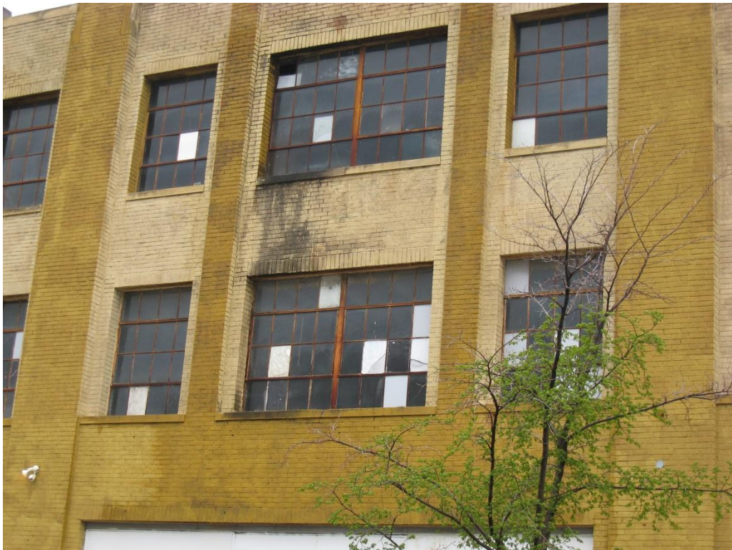
Deteriorated exterior walls, windows and paint at 4538 Troost Avenue (Deteriorated or inadequate site improvements)
