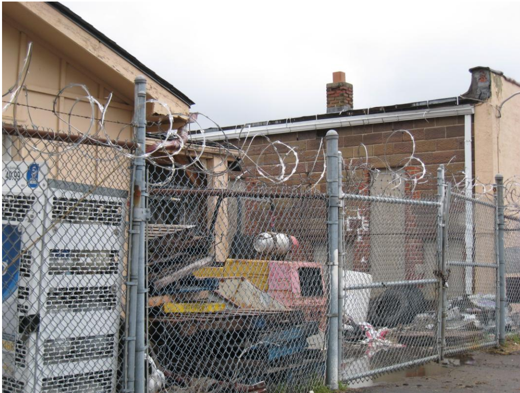
Accumulated debris and unsightly fencing rear of property at 4627 Troost Avenue ( Unsanitary or unsafe conditions, Deteriorated or inadequate site improvements )
