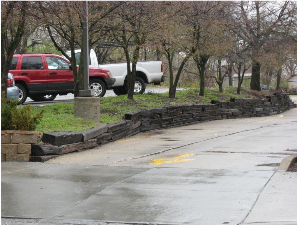
Deteriorated retaining wall and landscaping on north side of 1102 East 47th Street (Deteriorated or inadequate site improvements)
