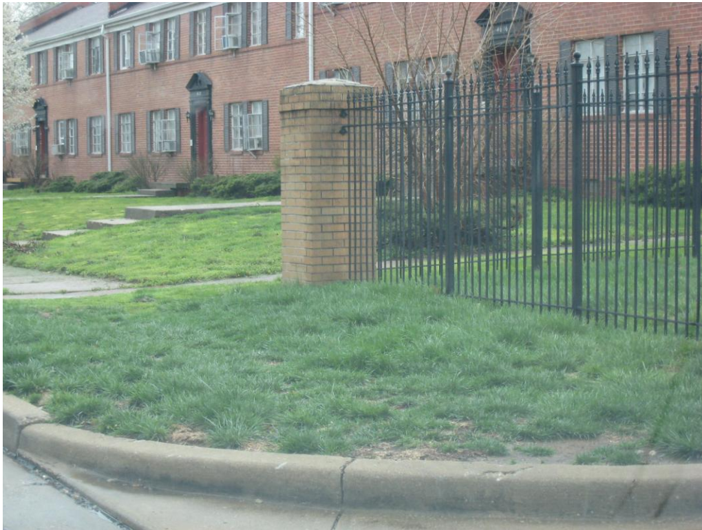
Lack of accessible public sidewalk, curb ramp east side 901 Brush Creek Boulevard (Deteriorated or inadequate site improvements)
