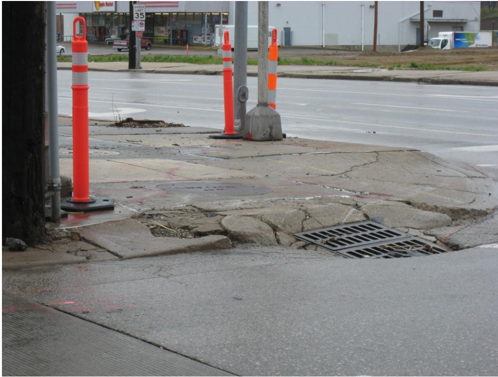
Storm water inlet at northeast corner of Troost Avenue and Emanuel Cleaver II (Deteriorated or inadequate site improvements)
