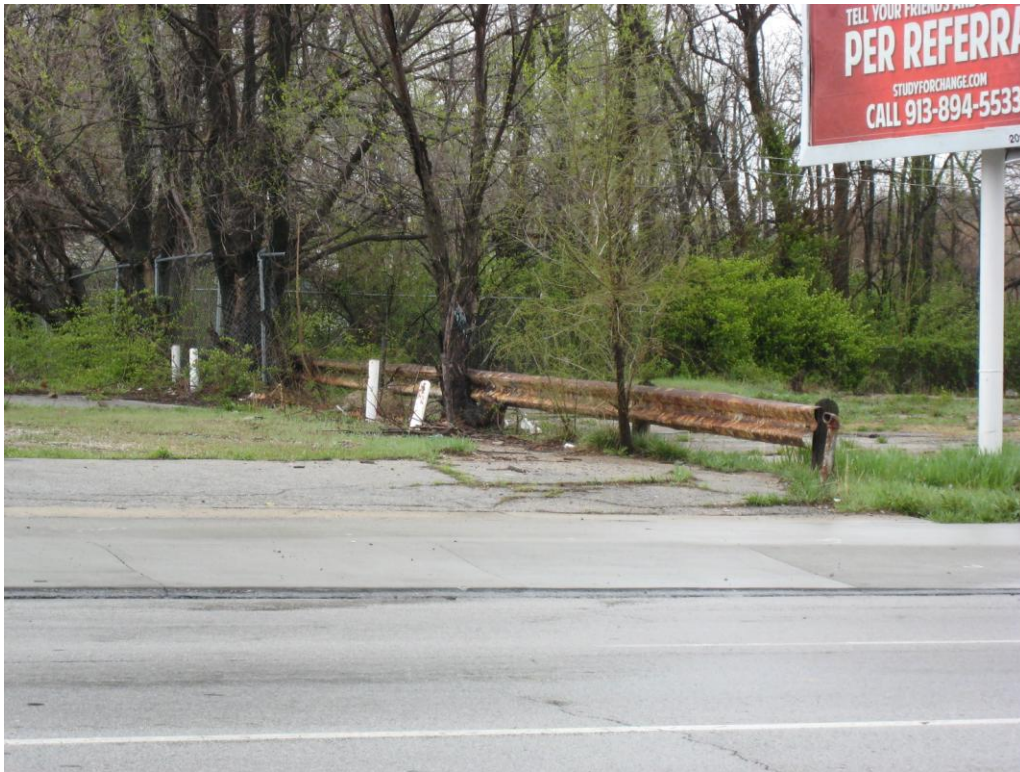
Deteriorated site conditions at southwest corner of property at 4601 Troost Avenue (Deteriorated or inadequate site improvements)
