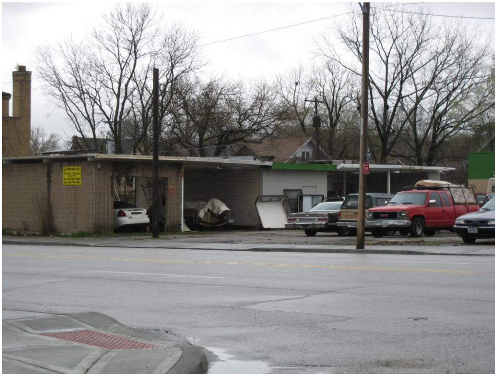
Poor building and site conditions, reuse of former carwash at 4504 Troost Avenue (Deteriorated or inadequate site improvements)
